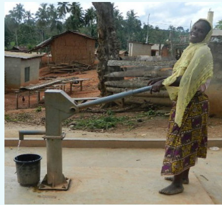
Local woman from Agona East using borehole and hand pump installed by USAID Ghana Mission and the Rotary Club of Tema. Photo by the Rotary Club of Tema
